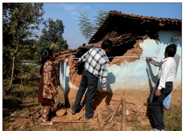
Figure 9. House damaged by elephants being assessed by government officials.
